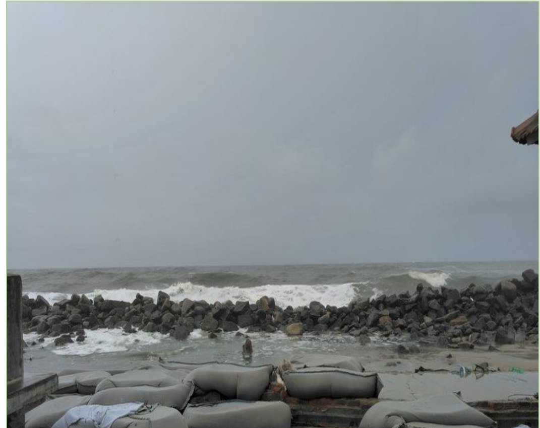
PICTURE OF SEAWALL BREACH IN KERALA
